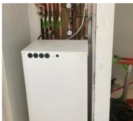
Figure 17 Example of residential Thermino heat battery installation 25
