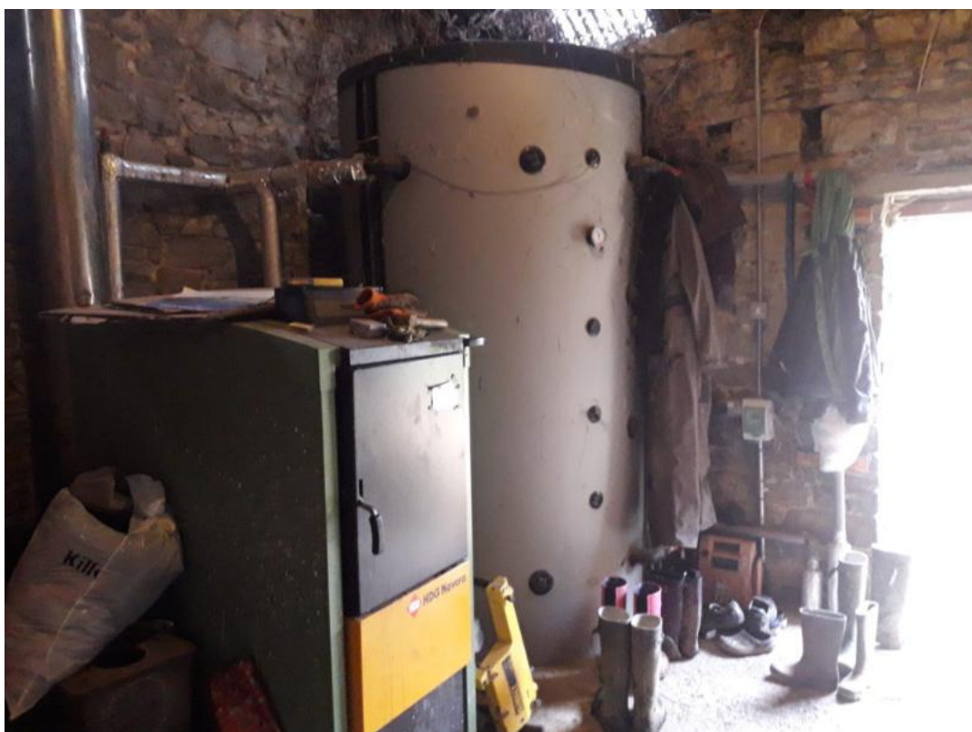
Figure 8: Glas Energy Case study: HDG Log Boiler system with 2000L buffer tank for Home Heating 9
