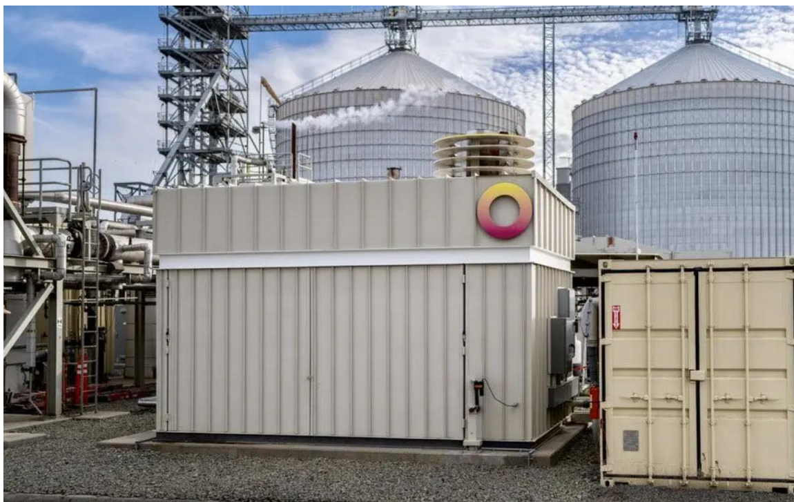
Figure 13: Rondo Heat Battery at Calgren Renewable Fuels facility 22
