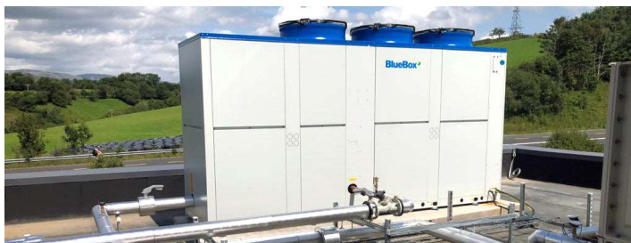
Figure 7: Swegon "Blue Box" Commercial Heat Pump
